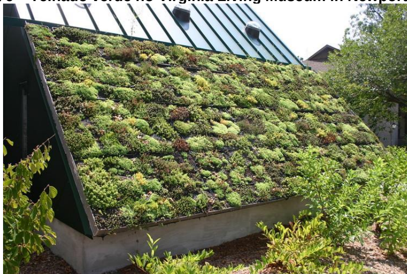
Figura 6 – Telhado verde no Virginia Living Museum in Newport News, Virginia
