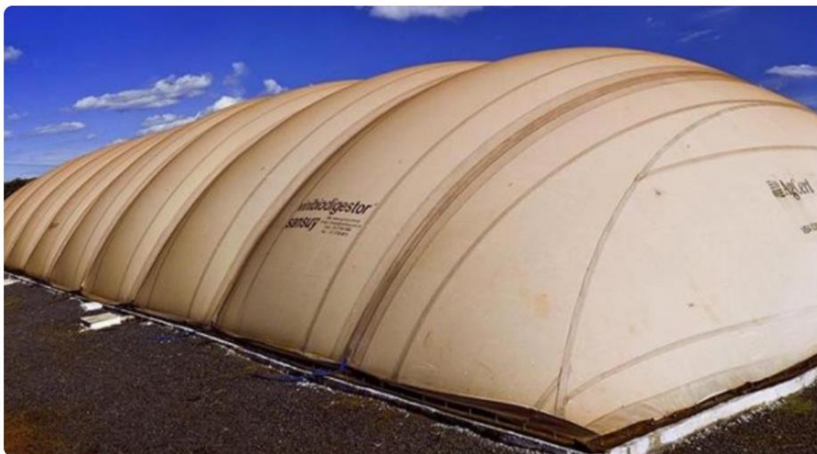
Figura 6 – Biodigestor Lagoa Coberta (BLC).
